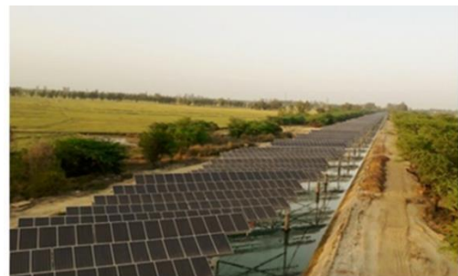
Figure 4. Ghaggar branch canal-top plant
